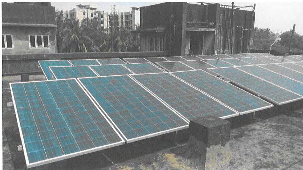
Photograph of Roof Top Solar PV Plant:
