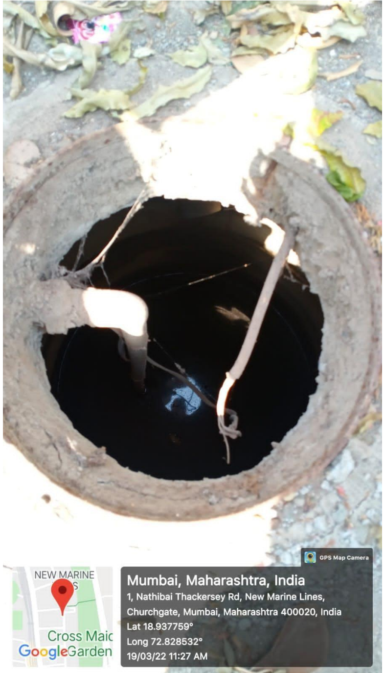
Rain water harvesting system at SNTWU, Churchgate Campus
