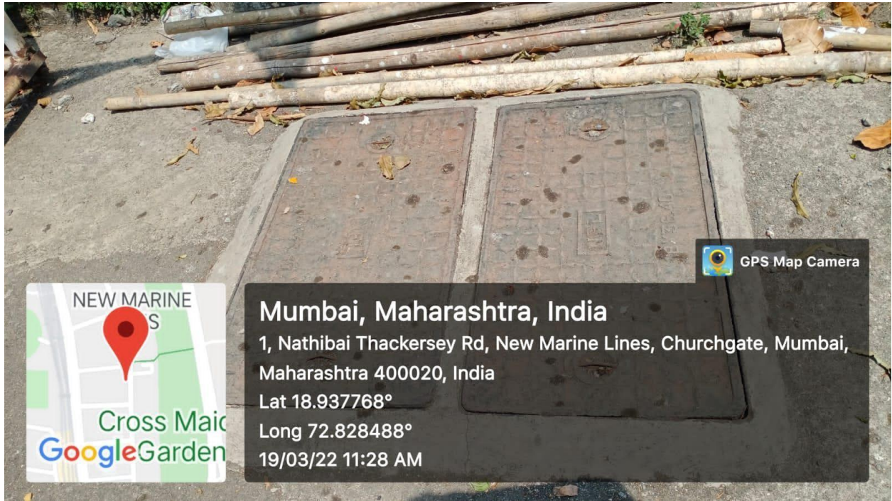
Rain water harvesting system at SNDTWU, Churchgate Campus
